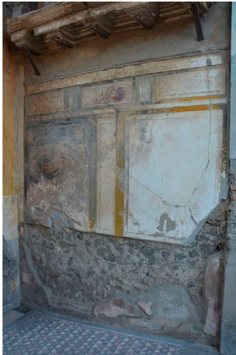
Figure 4. Casa del Fauno (VI 12), view from the western atrium toward the western wall of the fauces (7/53) (photo: Julika Steglich).
