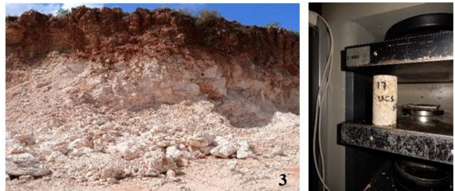
Figure 8. Litho3: Disintegrated high-grade rock is overlain with a layer of weathered rock/top soil. UCS = 5.24 MPa, n = 10.7\% , GSI = 17.
