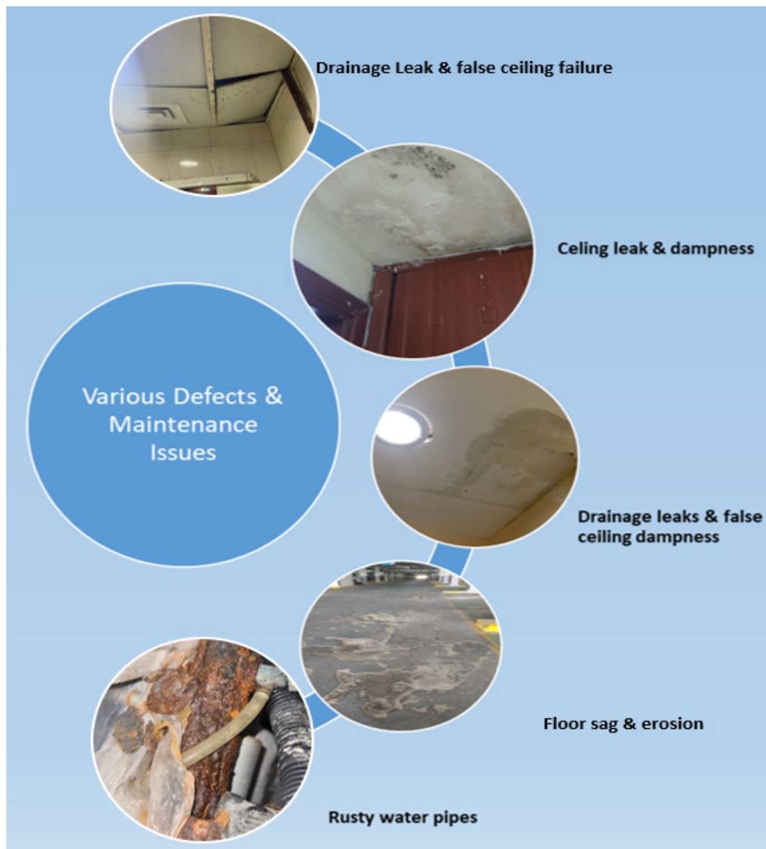
Figure 4. Different defects and maintenance issues.
