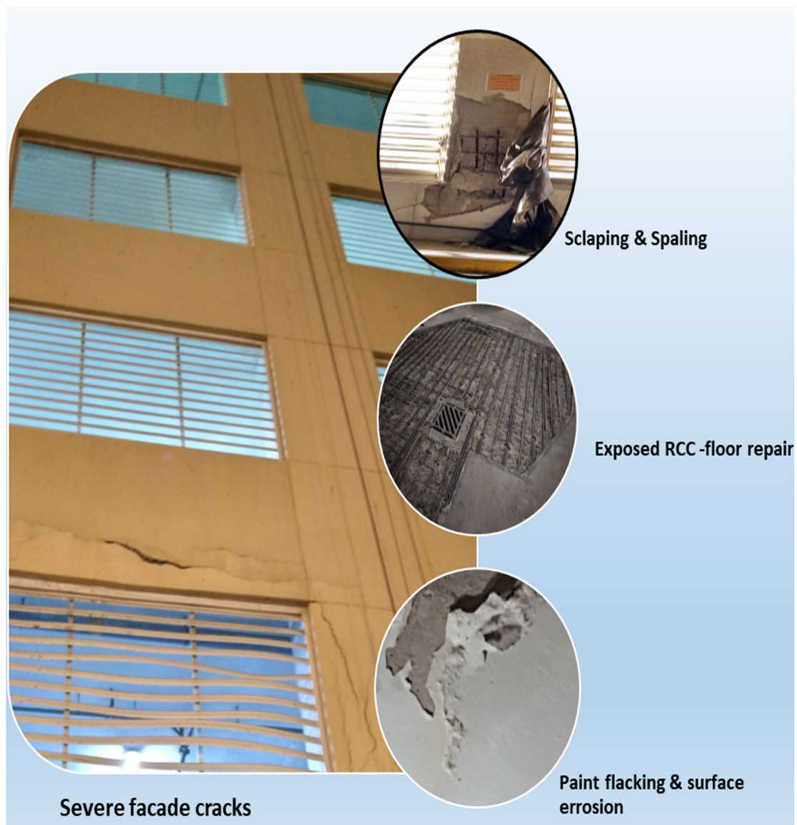
Figure 3. Construction and structural defects.
