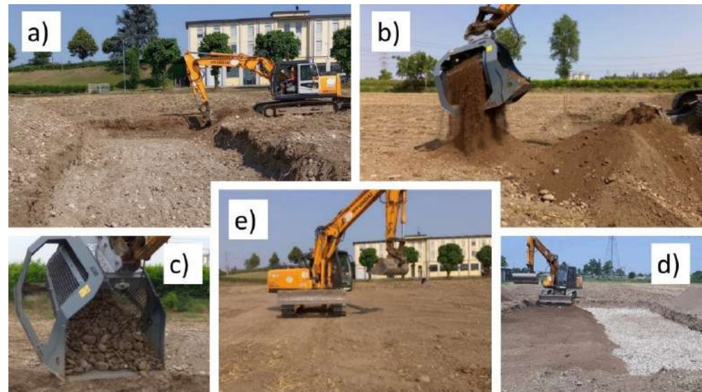
Figure 10. Scheme of the processing phase: (a) Trenches digging; (b) Soil sieving; (c) Discharging of retained stones in the trenches; (d) Refilling of trenches with sieved fine earth; (e) Compaction of sieved fine earth layer.
